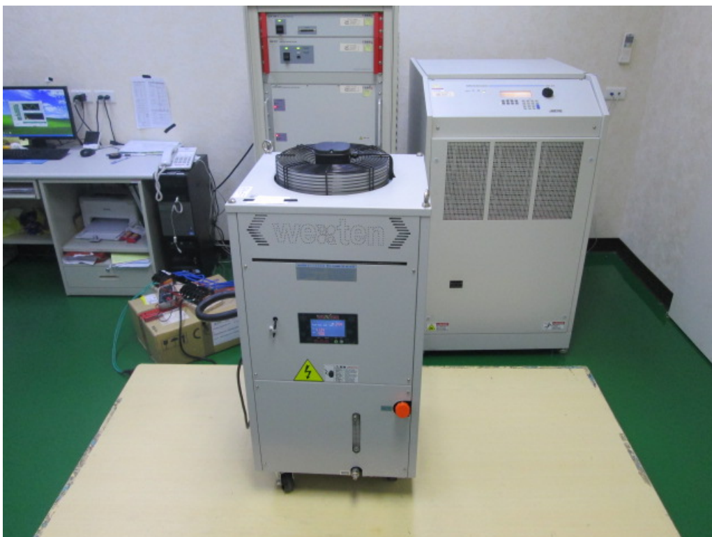
Picture 36: Test setup for Voltage Dips and Interruption, CWIDA12PTS (AC 400V)
